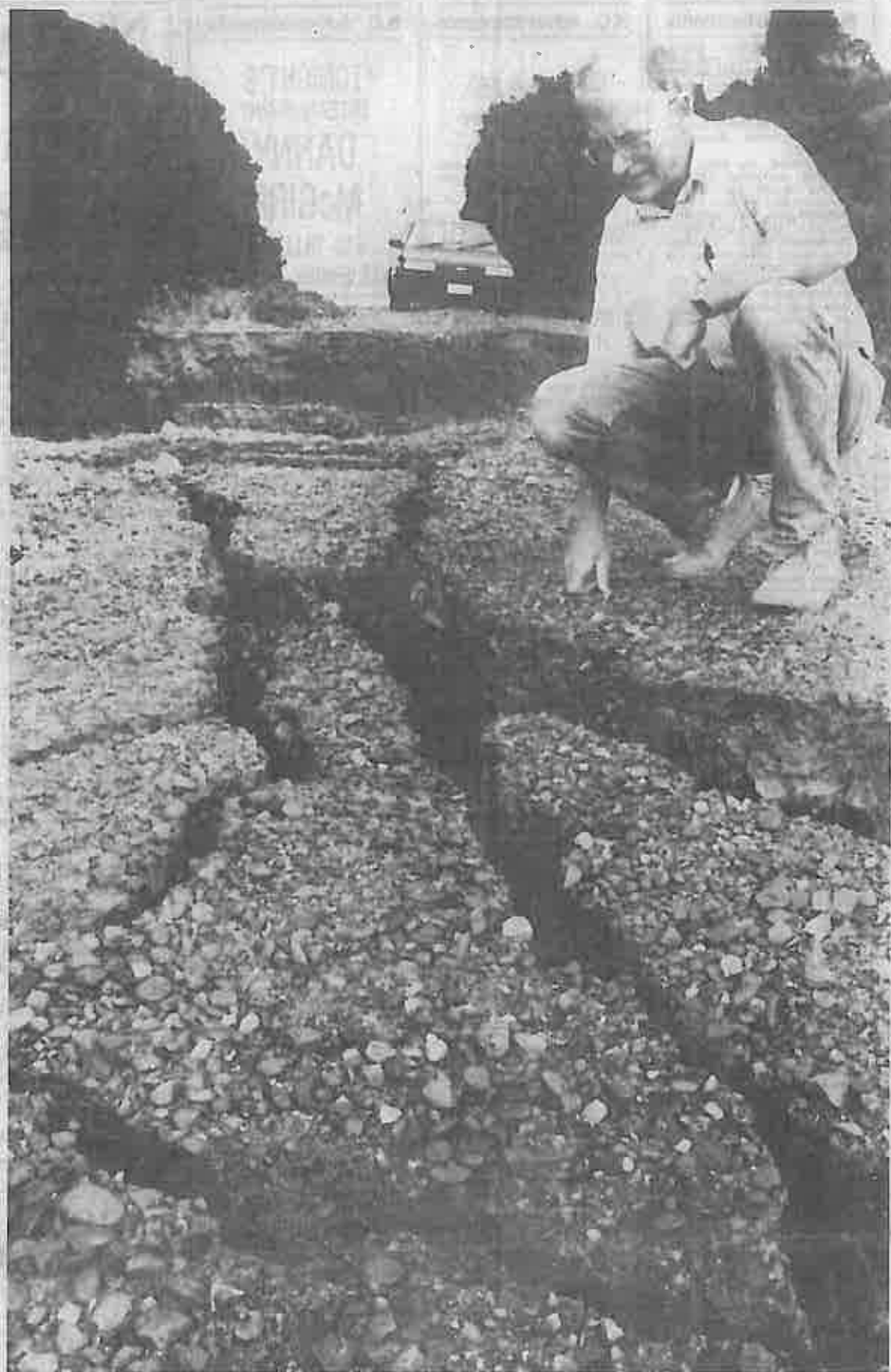
Mr Richard Hefford, an engineering seismology technical officer with the DSIR, examines subsidence in Virgin Flat Road near the epicentre of the earthquake near Westport on Tuesday morning. The road was reopened yesterday.
